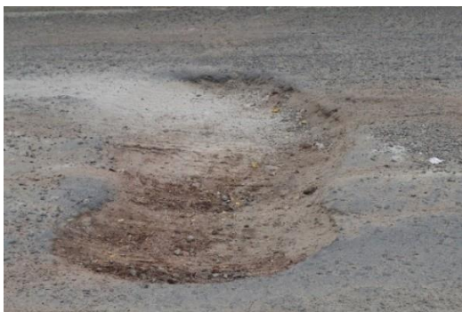
Figure 8 Potholes at Juni Vasti
