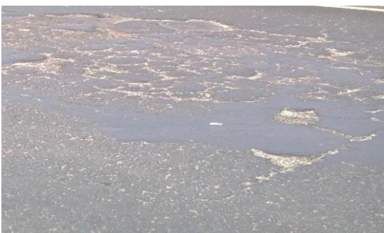
Figure 4 Block cracking at Laali Lawn
