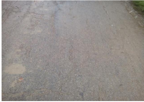
Figure 7 Longitudinal cracking at Yashoda Square
