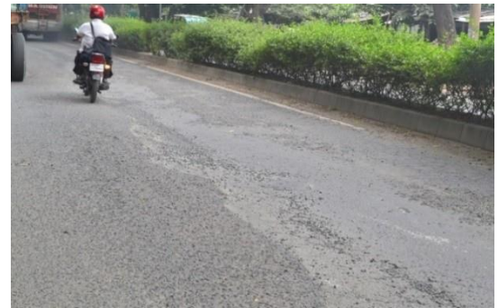
Figure 9 Raveling at Yashoda Square
