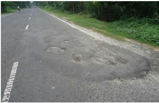
Figure 11 Corrugation and shoving at Dastur Nagar
