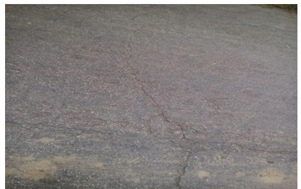
Figure 6 Transverse cracking at Dastur Nagar
