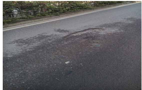
Figure 10 Water bleeding at Rayba Hotel
