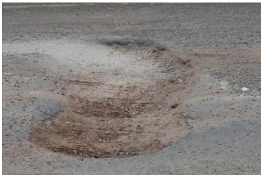
Figure 8 Potholes at Juni Vasti
