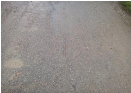
Figure 7 Longitudinal cracking at Yashoda Square
