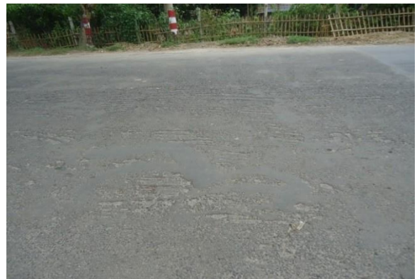
Figure 5 Slippage cracking at Chaprashhi Pura
