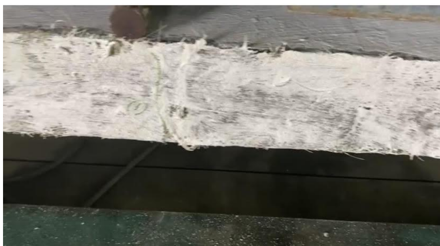
Fig 4.4.4: Cracked patterns on U wrapped collapsed beam after loading
