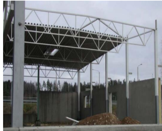
Fig- S-Market, Finland (Deconstruction and reassembly of a steel structure in a new location)
