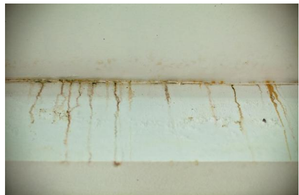
Fig Seepage through slab
