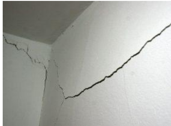
Fig cracks and damages
