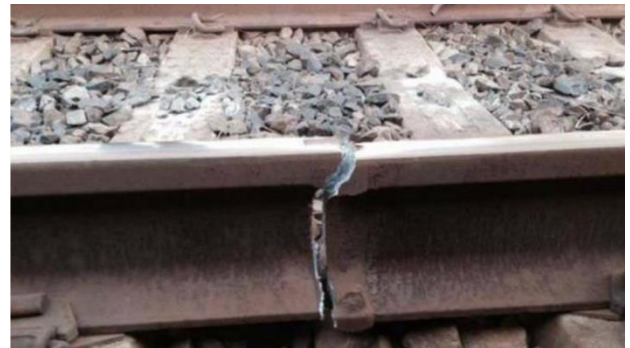
Figure 1 Wide crack on a running railway track [3].
