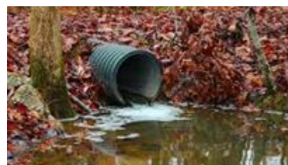
Fig -9: Liquid waste dispose to drainage
