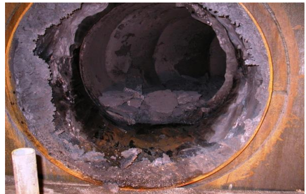
Fig -1: Fouling in chimney
