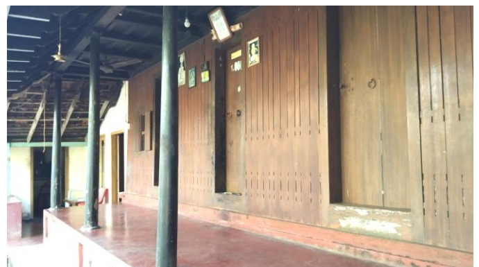
Fig -7: Verandah / open living space of Thevarpathiyil home (Original photo shot by Yadu Jagadish, inhabitant)
