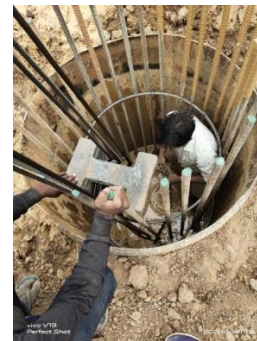
Figure 7: Construction worker entering rebar cage without any PPE and harness.
