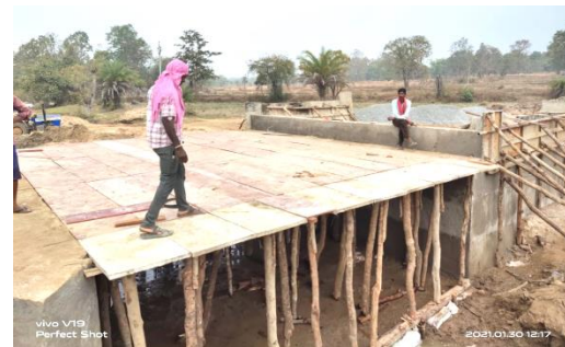
Figure 4: Working on a high level bridge without any PPE and harness to protect from falling
