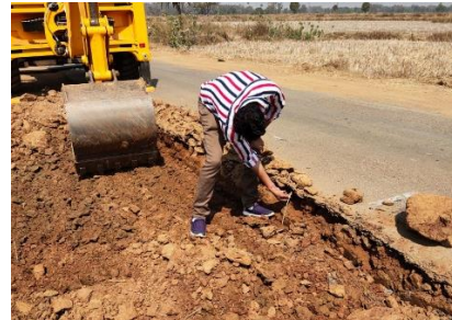
Figure 2: Perilous vertical cut
