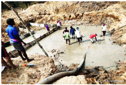
Figure 6: Construction workers exposed to wet concrete without any PPE and Foot protection (safety footwear, gumboots etc)
