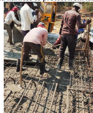
Figure 5: Construction worker working on an unstable platform
