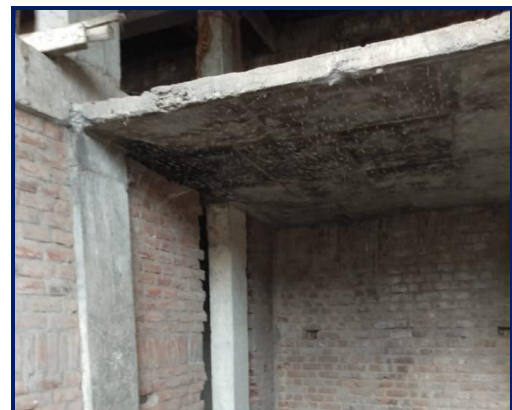
Fig -2: Visual Observation of Slab
