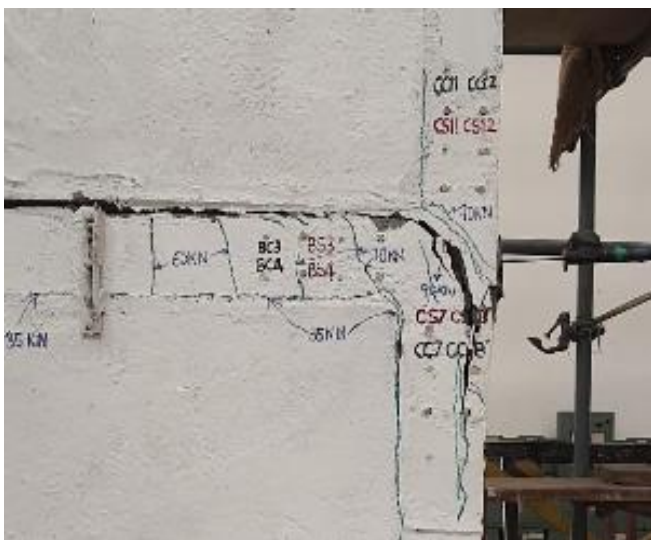
Fig -13: Joint failure
