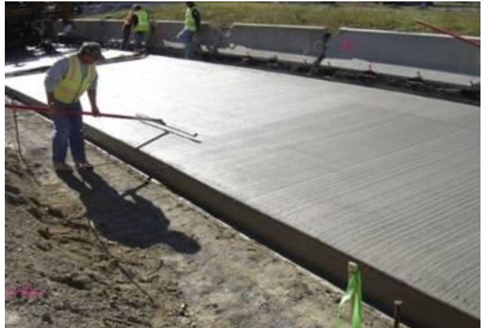
Fig No 3. Brooming of Rigid Pavement Surface
