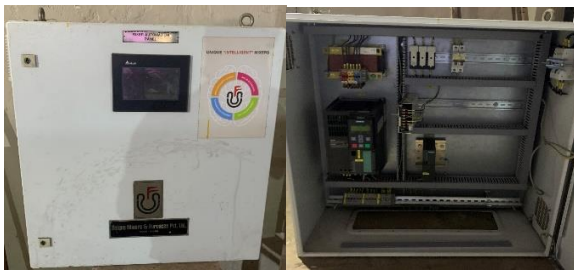
Fig 5. Automatic Control Panel
