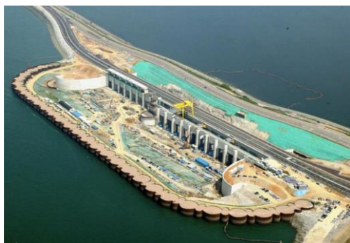
Fig-5: Sihwa Lake Tidal Power Plant
