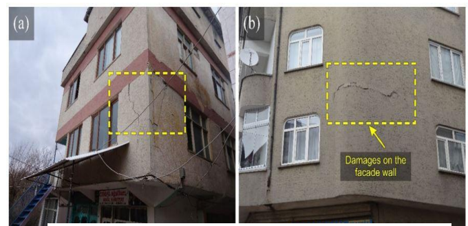
Fig. 1. Infill walls states after Sivrice earthquake in 2020
