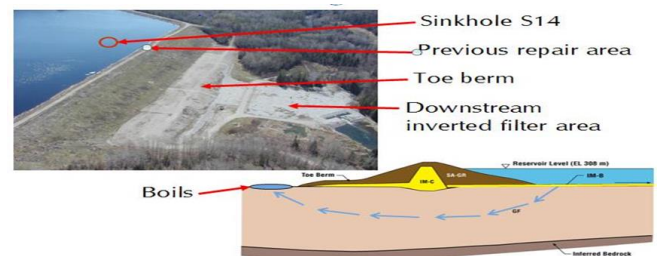
Fig -11: Shikwamkwa Dam: showing damage, filtered toe berm, and section of erosion pipes [9].
