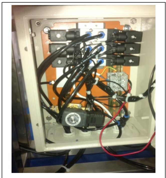
Figure.7 Control Panel for PPAR
