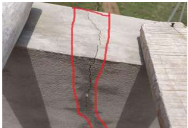
Fig 5- Crack on the Parapet wall
