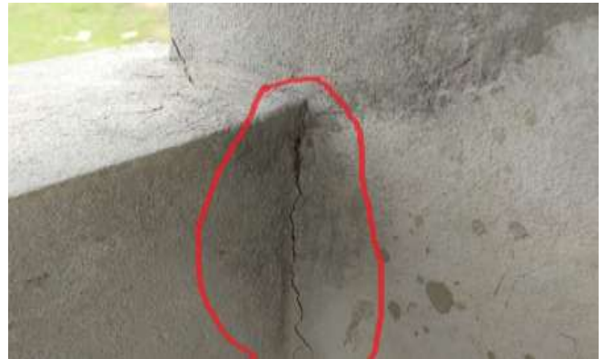
Fig -Crack at the corner
