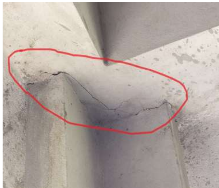
Fig 3 - Crack on beam and column junction.
