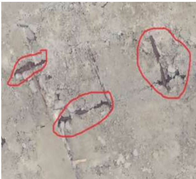
Fig 1 – Spalling of concrete slab.
