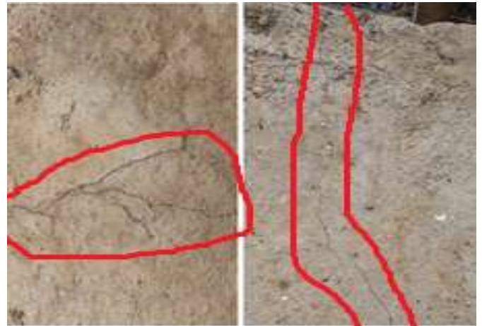
Fig 7- Cracks on slab.
