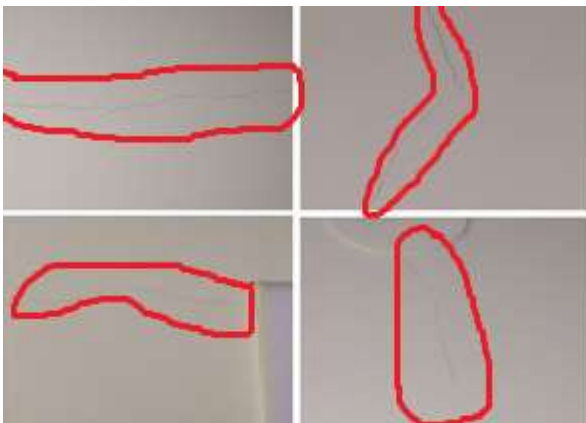
Fig 6-Hairline Cracks on Wall.
