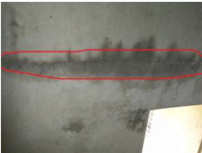
Fig 3- Horizontal crack on staircase.
