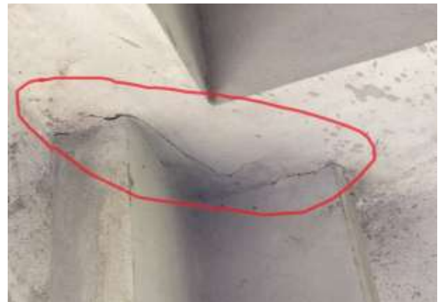
Fig - 1: Horizontal Crack at the beam-column junction.
