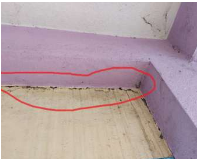
Fig - 3: Horizontal cracks in concrete wall.
