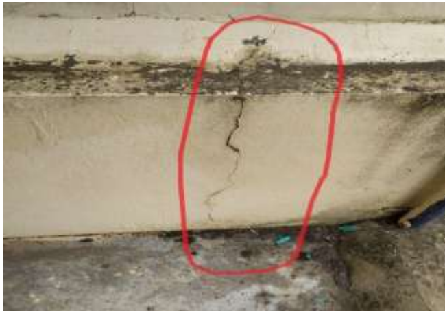
Fig - 2: Vertical cracks in concrete wall.
