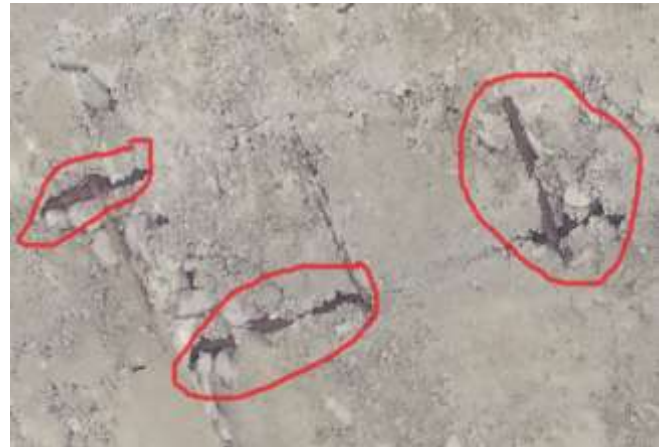
Fig-7: Improper reinforcement on slab.
