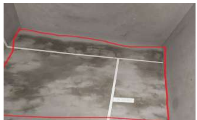
Fig - 5: Moisture defects on wall.
