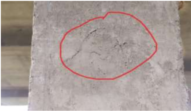
Fig – 6: Cracks in Concrete Columns
