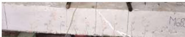
Fig-19: Crack pattern of B3 type beam
