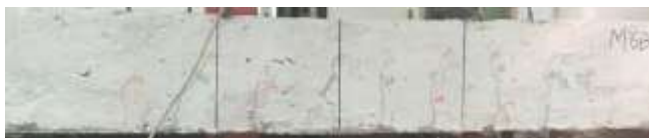
Fig-18: Crack pattern of B2 type beam
