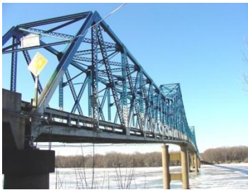
Figure-6: Coated Bridge structure for protection against corrosion
