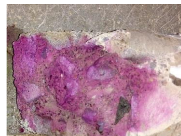
Fig -1: Carbonation test sample of Beam 02
