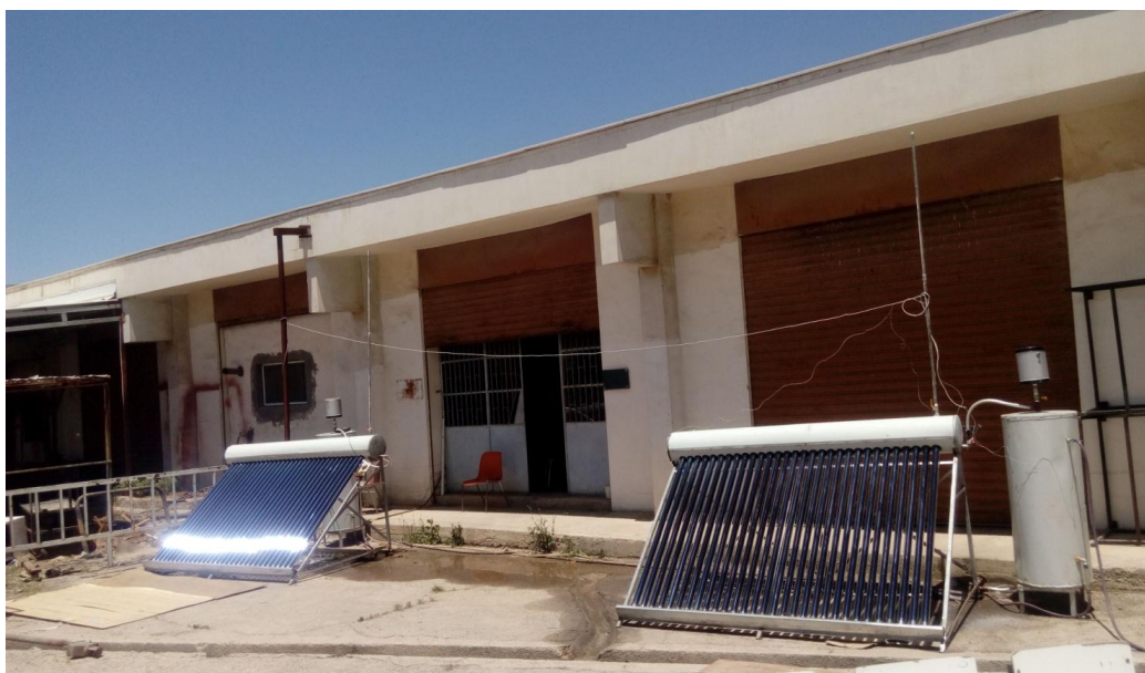
Fig. 3.2 Two identical evacuated tube solar water systems with indirect storage tank.
