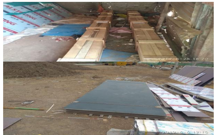
Wastage of ACP material, poor
