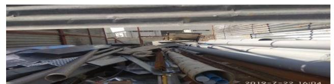
M.S materials are thrown on PVC plumbing materials due to pipes are damaged
