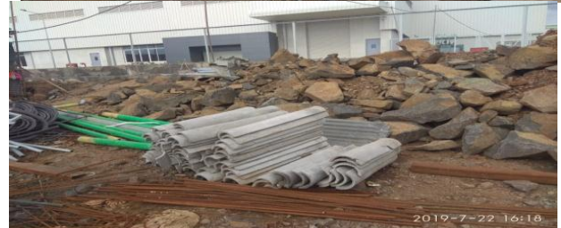
Poor storage of RCC Hume pipes
