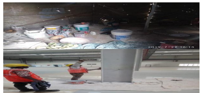
Wastage due to bad storage & Wastage due to rework
