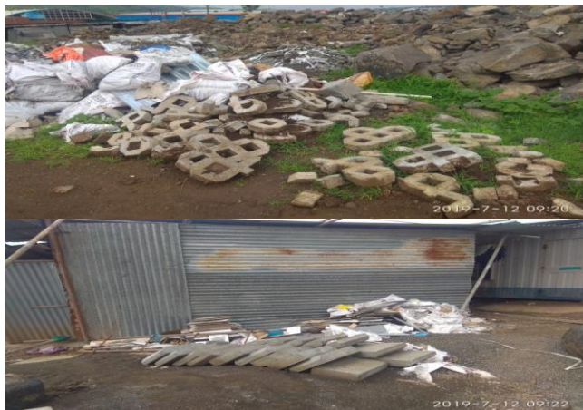
Damages to paver block due to handling Damages to kerbs due to bad storage
