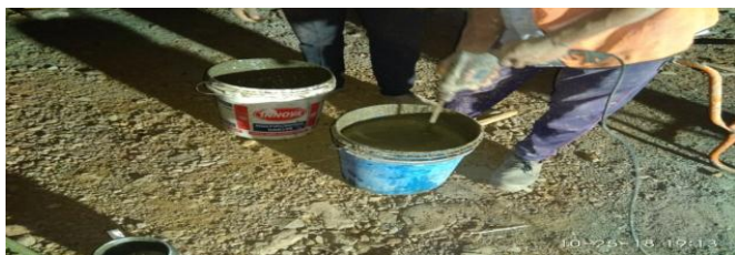
Wastage due to poor handling Wastage at time of mixing and placing
