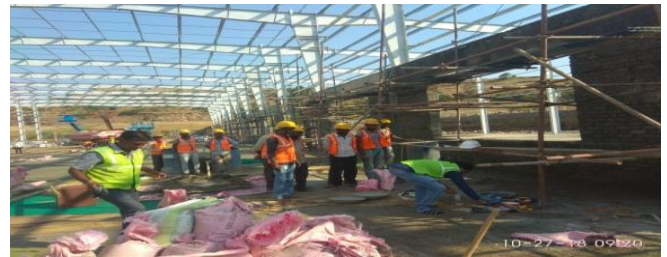
Wastage due to rework of wall - plaster
