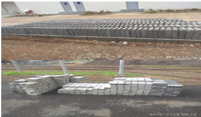
Kerb stones and paving blocks to be stored on leveled ground to avoid sliding
