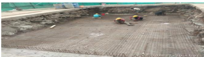
Wastage of steel due to poor storage Wastage due to replacement
