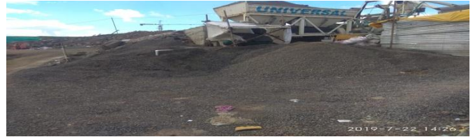
Wastage of aggregate due to improper handling and storage on batching plant
