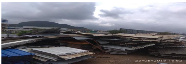
Wastage due to bad handling and storage
