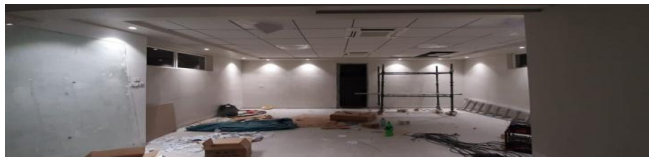
Wastage due to bad workmanship Damages to painted
