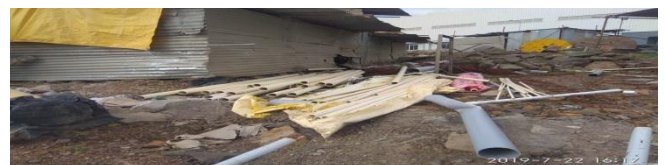
Plumbing materials are thrown in steel yard, poor handling a
