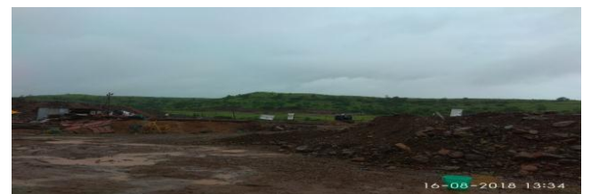
Wastage due to keeping expose in rain
