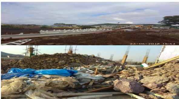
Steel wastage due to bad storage
