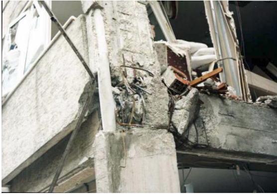
Photograph -1: Damaged beam-column joint during earthquake (Kocaeli, Turkey 1999) [5]
