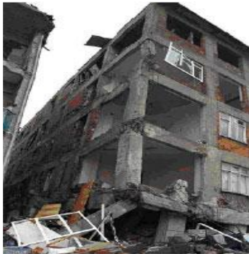
Photograph -2: Beam-column connection failure, Izmit, Turkey, 1999 earthquake [5]
