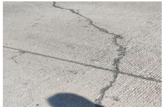
Fig -1: spalling on pavement
