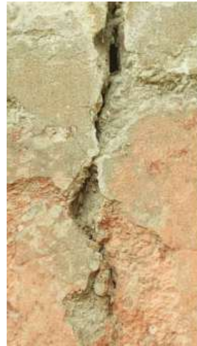
Figure 2 Cracks at Plinth Level
