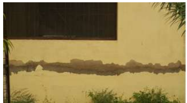
Figure 3 Seeping of water at plinth level due to high water table
