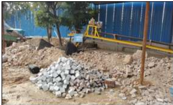
Fig -1: Collection of waste on site
