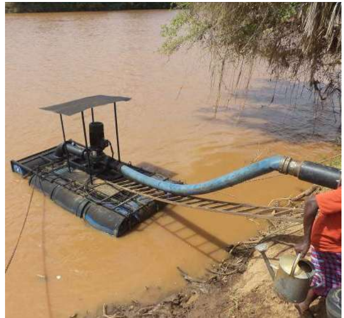
Figure -7: Pump and the pump system installed on site
