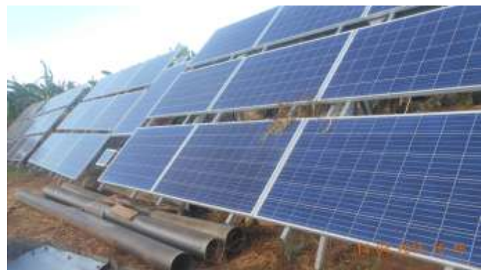
Figure -8: Photovoltaic modules on site
