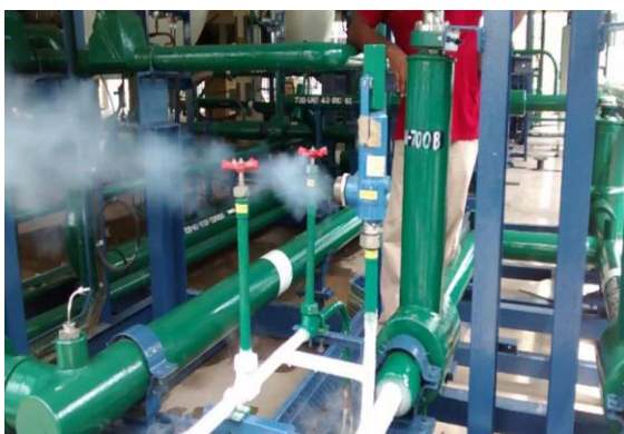
Fig 2.1: Cryogenic PRV in operation at LSSF
