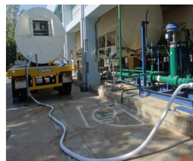
Fig 4.2: Liquid nitrogen storage tank at operation
