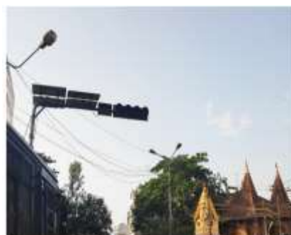
Fig -9: Signals are not in working condition
