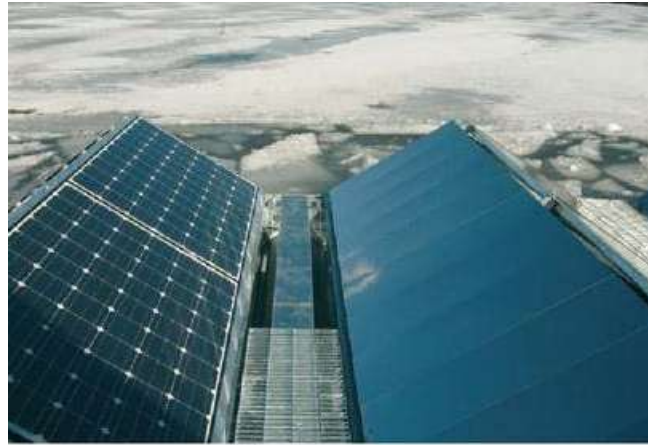
Fig. 6. 20kWp FTCC System in Cheogji, South Korea with can withstand water freezing temperatures
