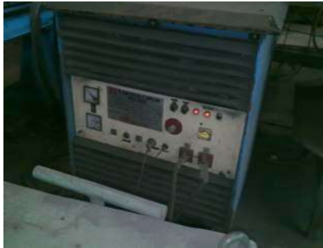
Fig. DC Power Supply Source
