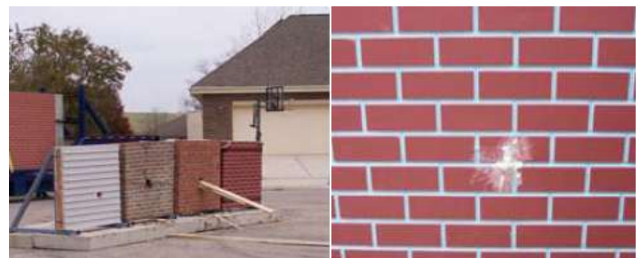
Figure 5 shows damage of wall against tornado
