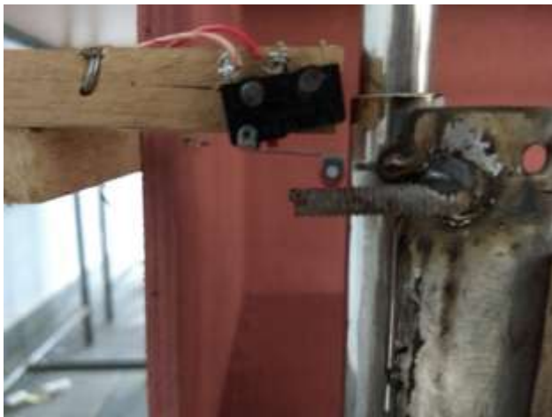
Fig - 11 Limit Switch being triggered
