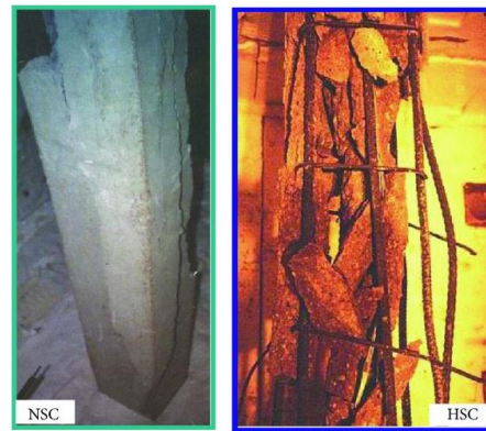
Fig -2 : HSC and NSC column after fire [13]
