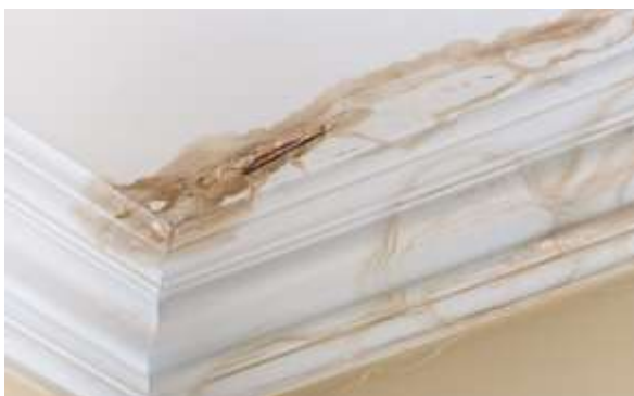
Fig-3: - Water Effect in Inside Plaster
