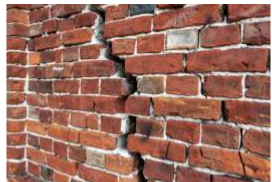
Fig-4: - Cracking in Brick Work
