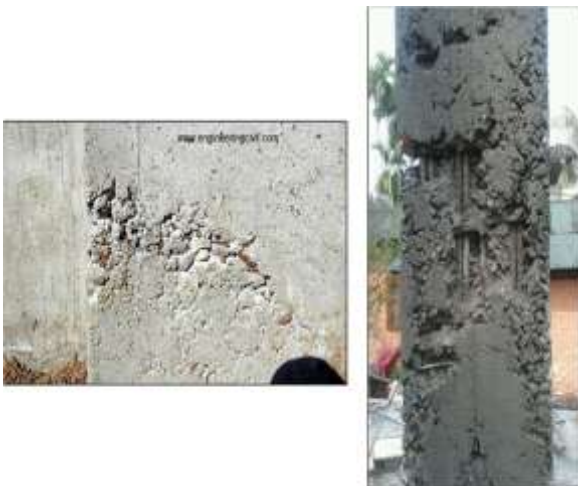
Fig -1: -Honeycombing in Column
