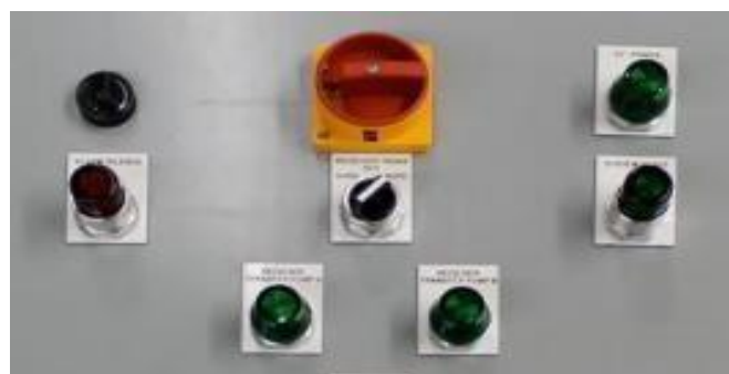
Fig.15 A Simple Control Panel with Push Buttons and Switches with Indicator Lights
