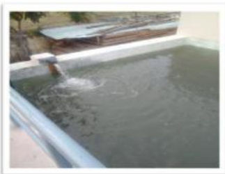
Fig. 2.4 Effluent after treatment, (Treated effluent collection tank).
