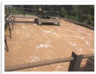
Fig. 2.3 Effluent under treatment, (Aeration tank).
