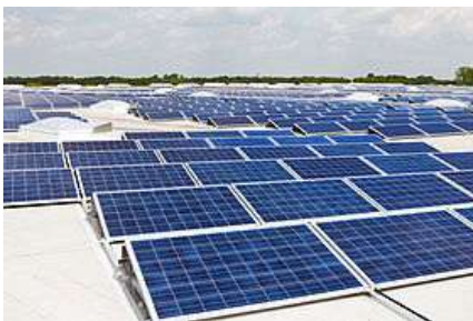
Fig -2.1: Solar Panel
