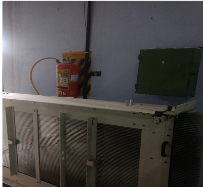
Figure 4.1 Extinguisher in unaccessible area
