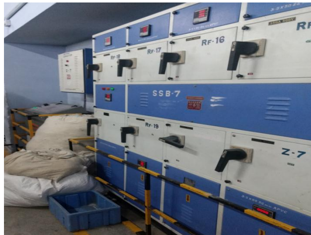
Figure 3.1 Stacking flammable material near panel board
