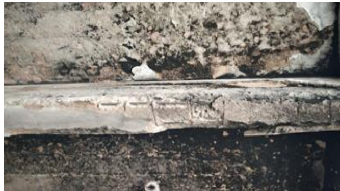
Figure: 1. Concrete Structure After Exposure to Fire.
