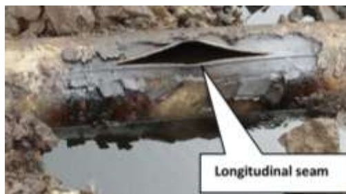
Figure 3b: Preliminary failure photographs at site
