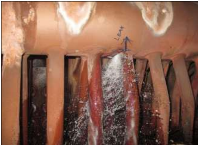
Image 2 Failure of tube and pipe joint
