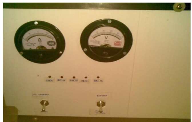
Fig-11: The bottom half view showing the meters, switches & LEDs
