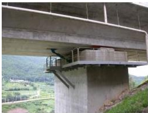
Fig -1: Damper installed in Ok-yeo bridge
