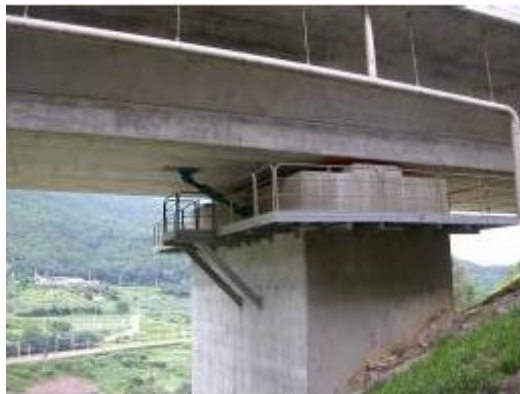
Fig -1: Damper installed in Ok-yeo bridge
