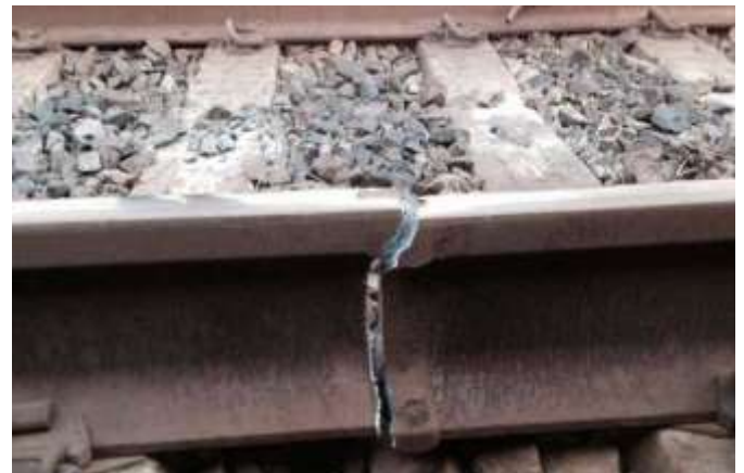
Fig -1: Cracks on railway tracks
