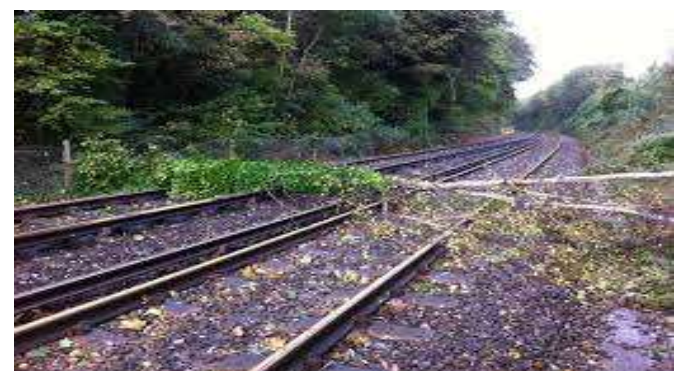
Fig -2: Tree fallen on the railway tracks
