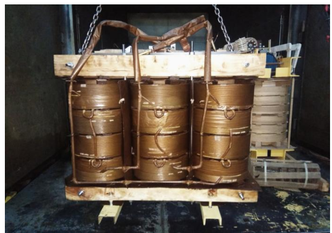
Fig -2: Transformer with wooden clamping
