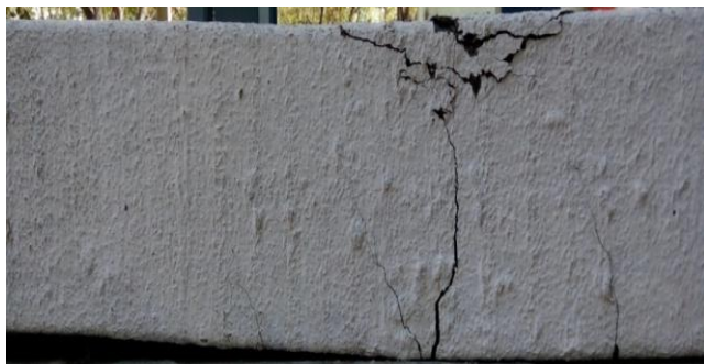
Fig 4.5 Crack pattern of control beam
