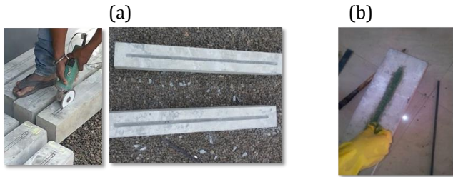
Fig -4: (a) Cutting of grooves and (b) filling of grooves with epoxy
